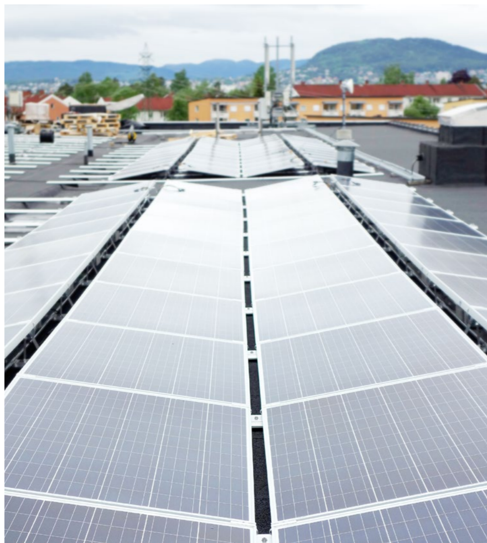
In May 2016, 180 solar panels were installed in KONE Oslo's passive energy house covering one third of the rooftop.
